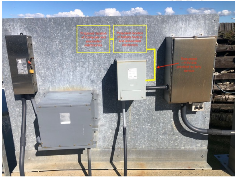
Figure 1: Proposed placement on existing power station.
